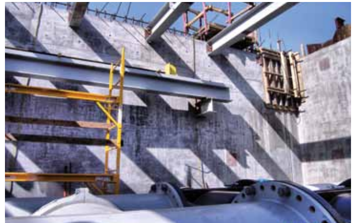
Installation of beams for an overhead travel crane at Bitter Point Pump Station. The crane is used for maintenance or repair purposes.
