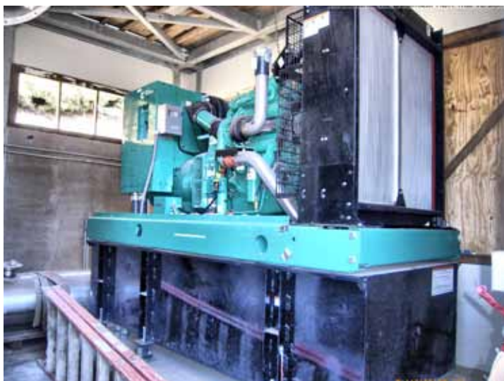
Stand-by generator for the Rocky Point Pump Station is used to keep the station running in the event of electrical outage.
