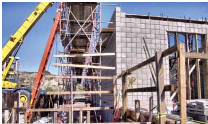
Construction of the masonry walls for the electrical building for the Bitter Point Pump Station.
