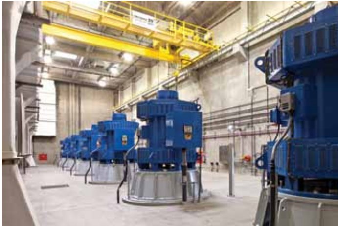
The Headworks Improvement project replaced the influent pumps with new 700 hp pumps capable of raising the water almost four stories to allow treatment.
