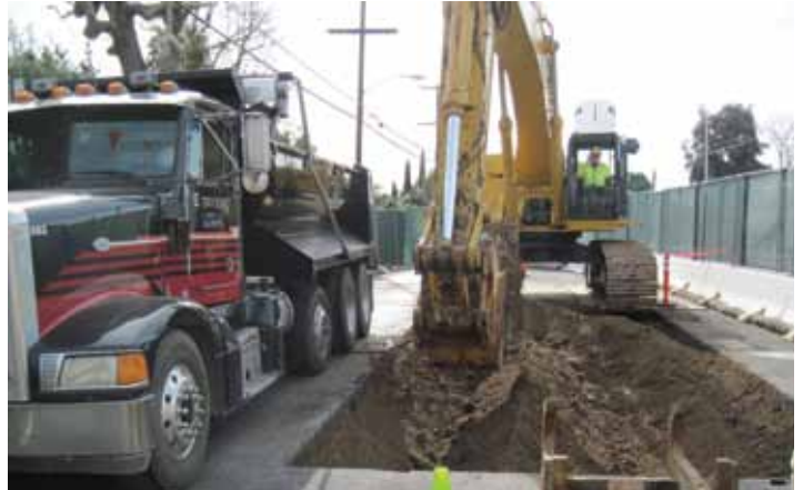
Excavation of installation pits allows existing underground piping to be rehabilitated in OCSD's design-build project.
