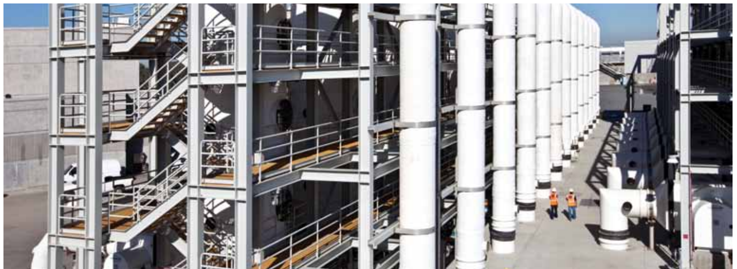
The new state-of-art odor control system at Plant No. 2 uses biofilters to clean the air and save on chemical costs.
