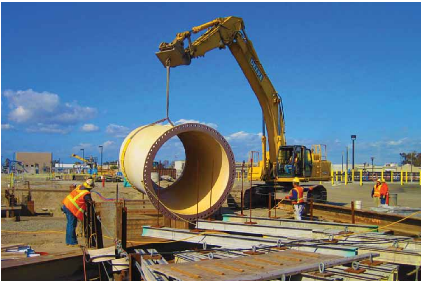
Installation of new 90-inch secondary effluent pipeline in the P1-102 Secondary Treatment Facilities at Plant No. 1.
