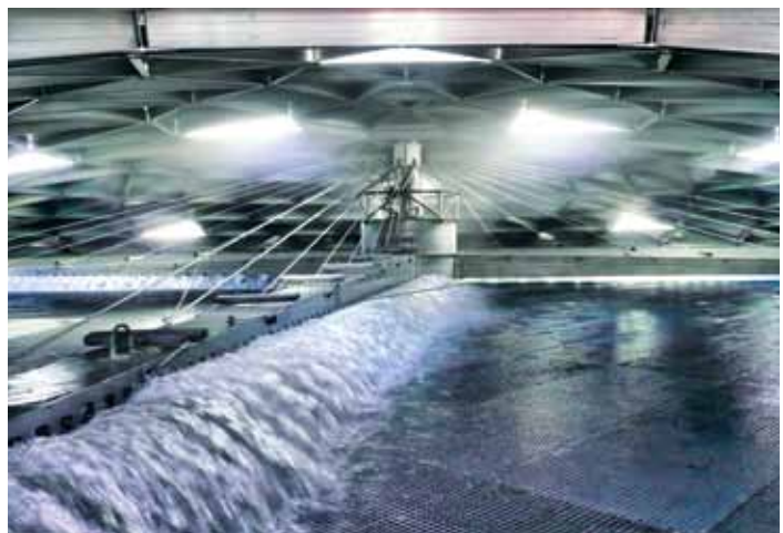
Recently completed Trickling Filter at Plant No. 2 which is now in service.
