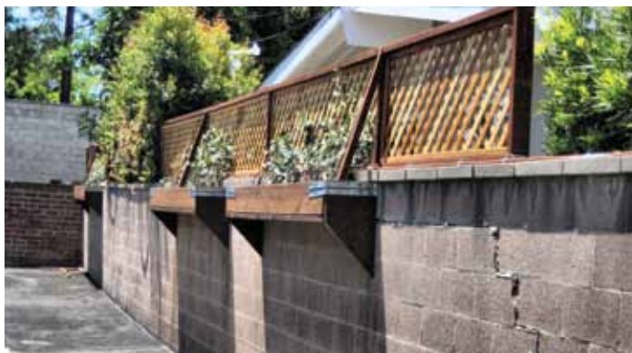
At our Westside Pump Station, landscaping was added along the perimeter walls of the property to screen views of the pump station from neighboring homes.
